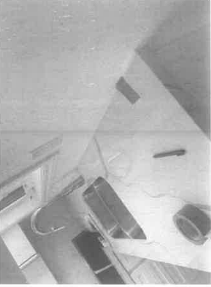
173301 - 2 - COUNTERTOPS~COUNTERTOP RIGHT OF SINK NOT FLUSH WITH WALL.
