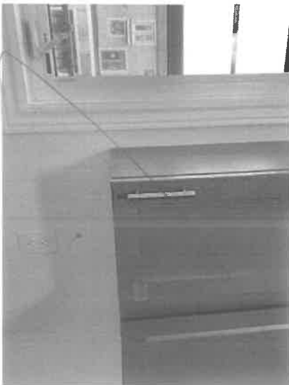
169698 - 1 - CABINETS~CHIP AT UPPER RIGHT CABINET RIGHT OF SINK
