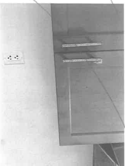
169697 - 1 - CABINETS~CHIP AT UPPER RIGHT CABINET LEFT OF HOODFAN.
