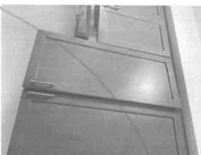
169695 - 1 - CABINETS~ADJUST UPPER LEFT CABINET RIGHT OF HOODFAN
