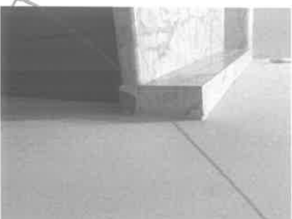
169689 - 1 - COUNTERTOPS~CHIP AT RIGHT EDGE AT SIDE SPLASH.
