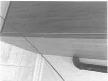
169685 - 1 - NOTE:~CHIP AT RIGHT GABLE.
