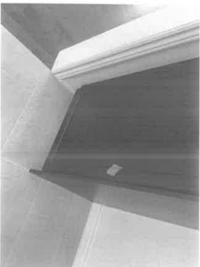
168097 - 1 - CABINETS~DENT ON PANTRY DOOR LEFT OF FRIDGE
