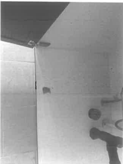
168095 - 1 - CABINETS~DAMAGE BOTTOM GABLE BELOW SINK AT ISLAND.
