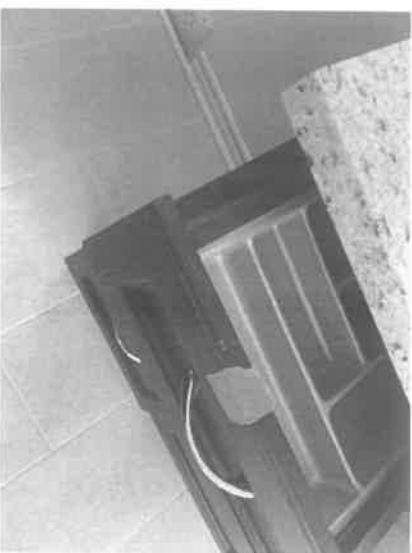
168096 - 1 - CABINETS~CHIP AT 1ST BANK OF DRAWER RIGHT OF STOVE
