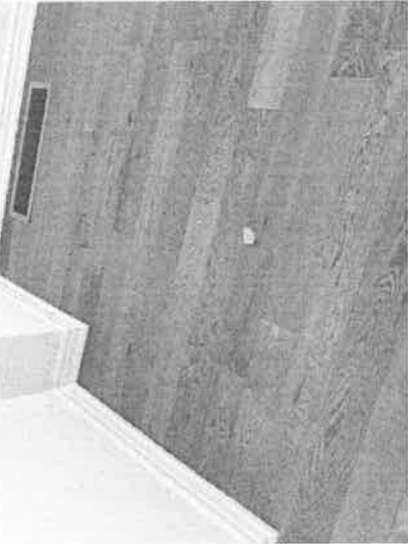
CORNER WALL INFRONT OF INTERNET ROUGH IN 4)CHIP ON 4RTH HARDWOOD PLANK INFRONT OF FIRE PLACE 5) INSPECT FILLER USED AT HARDWOOD INFRONT OF WINDOW
