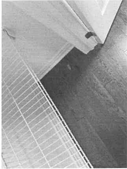
153629 - 2 - FLOORING~SCRATCH AT 2ND PLANK RIGHT SIDE INSIDE LINEN CLOSET 2) SMALL CHIP AT FIRST HARDWOOD PLANK BY NOSING AT STAIRS TO MAIN FLOOR LEFT SIDE
