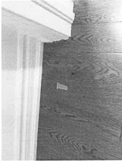
153629 - 1 - FLOORING~SCRATCH AT 2ND PLANK RIGHT SIDE INSIDE LINEN CLOSET 2) SMALL CHIP AT FIRST HARDWOOD PLANK BY NOSING AT STAIRS TO MAIN FLOOR LEFT SIDE
