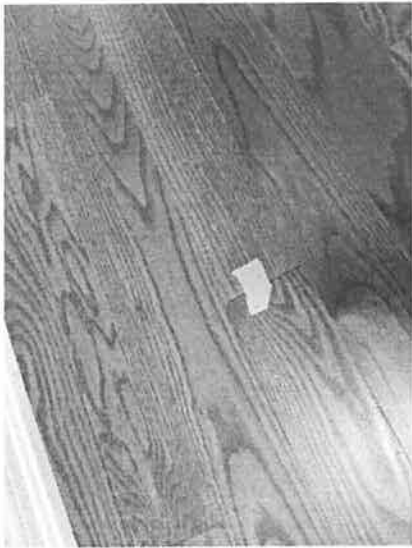
154870 - 1 - FLOORING~GAP AT 4 PLANK FROM ELECTRICAL OUTLET RIGHT OF 2ND BED ROOM BETWEEN TWO PLANKS
