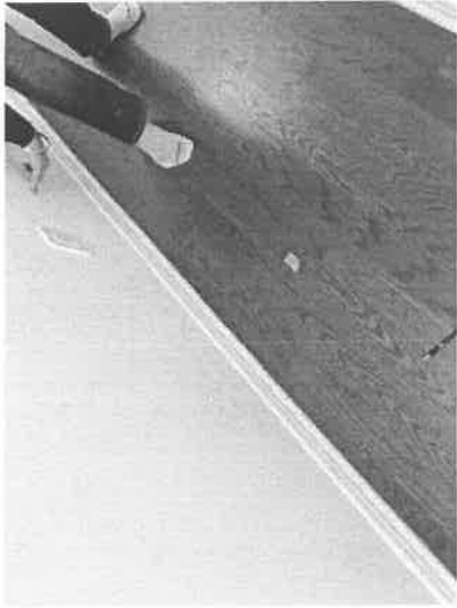
154870 - 2 - FLOORING~GAP AT 4 PLANK FROM ELECTRICAL OUTLET RIGHT OF 2ND BED ROOM BETWEEN TWO PLANKS
