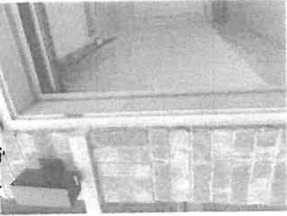
151596 - 1 - PORCH-PAINTING NOT COMPLETE AT GARAGE DOOR TRIM
