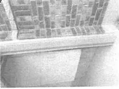
151596 - 2 - PORCH-PAINTING NOT COMPLETE AT GARAGE DOOR TRIM
