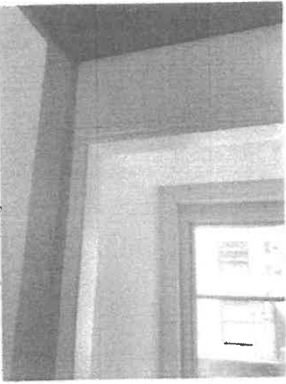
154570 - 2 - WALLS~INSPECT PAINT AT TRIM ARCH WAY AT ENTRANCE TO LIVING ROM FROM KITCHEN RIGHT SIDE
