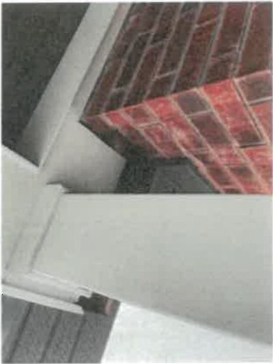
153252 - 1 - BRICKS--BRICK REQUIRED AT UPPER RIGHT GARAGE DOOR BY SOFFIT
