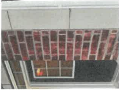
153310 - 1 - NOTE:--HOMEOWNER UNHAPPY WITH CUTS OF BRICK ESPECIALLY RIGHT SIDE OF FRONT DOOR
