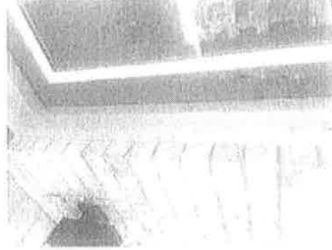
148826 - 1 - 1 - Dent on left door jamb at exterior
