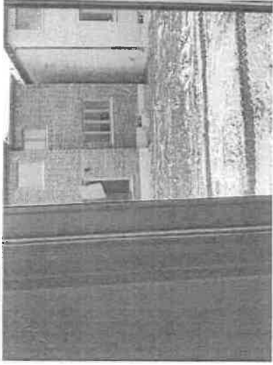
152290 - 1 - WINDOWS~CIRCLE CRACK ON LEFT FIXED WINDOW
