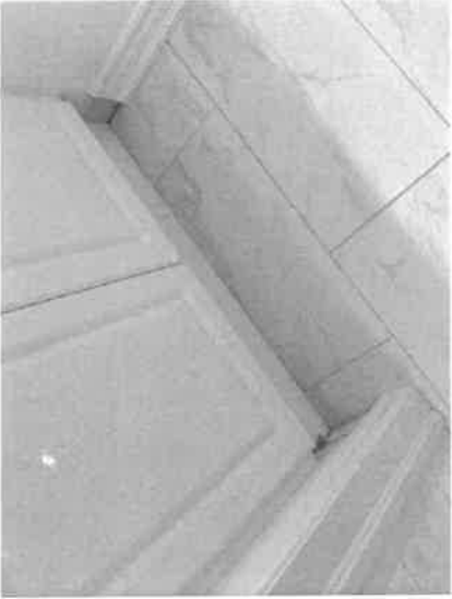
151161 - 1 - TRIM~MISSING TRIM RIGHT AND LEFT OF VANITY
