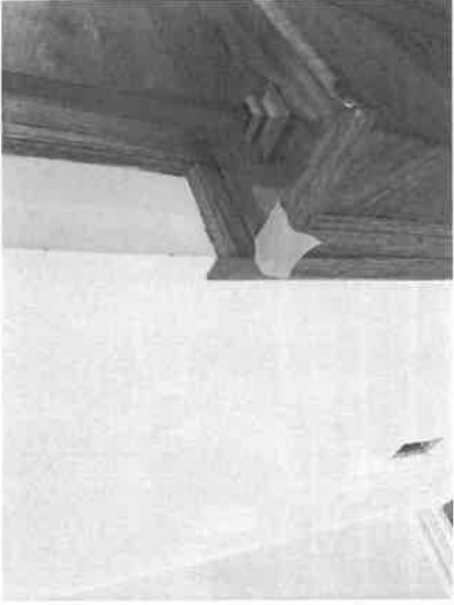
151223 - 1 - STAIRS~GAP BETWEEN TRIM AND TREAD AT STAIRS TO SECOND-FLOOR FIFTH TREAD
